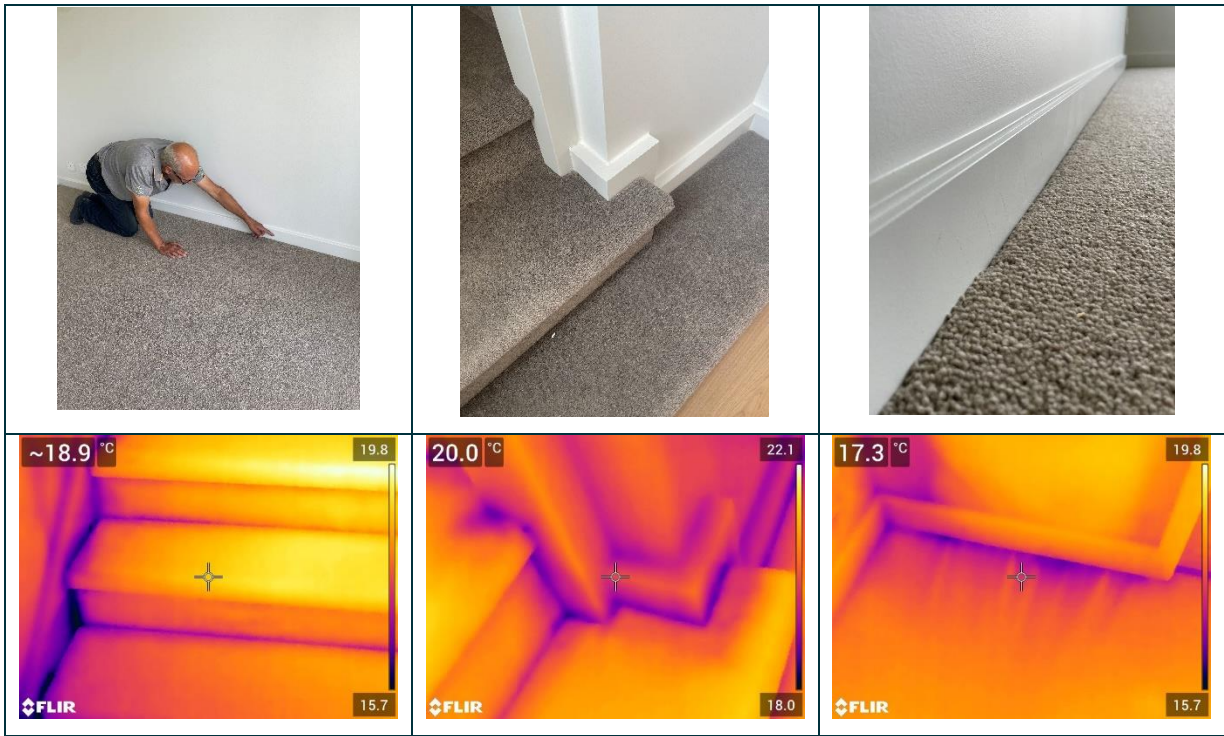
Figure 51 Examples of leakage points identified, but too difficult to measure
