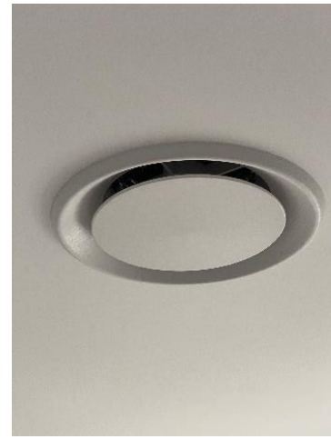
Ceiling vent with remote in-line fan
