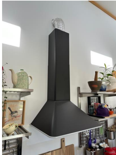
Ducted through wall
