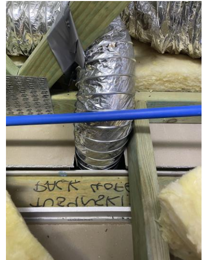
Duct through ceiling – note removed insulation
