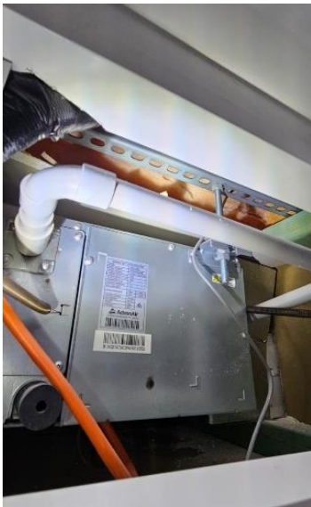
Insulation visible above unit, showing poor isolation
