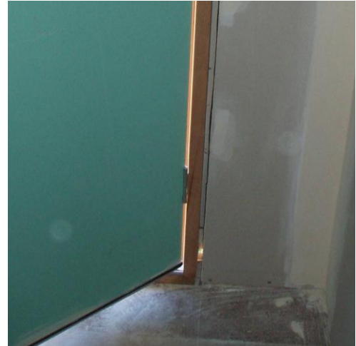
Figure 2.30 - Daylight is visible at the base of the gap between door jamb and wall frame
