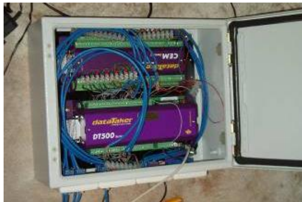
Figure 3.54 - Data-logger within a steel security box to eliminate effects from air movement
