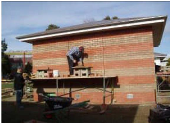
Figure 2.19 – Bricklaying completed with expansion joints in the wall for the knock-out panels (July 7, 2006)
