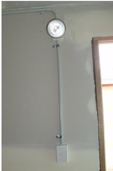
Figure 2.35 - Detail of surface mounted lamp and lamp switch
