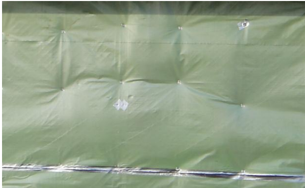
Figure 2.52 - Billowing of building wrap as a result of insulation installation
