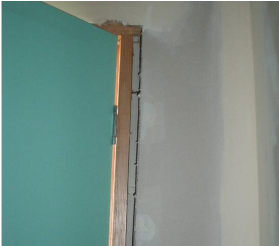
Figure 2.29 - Gap between door jamb and wall frame is clearly visible
