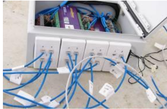
Figure 3.4 - Analogue data-logger as installed in the test cell (July 2006)
