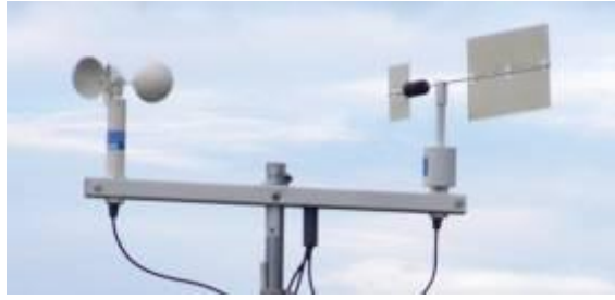
Figure 3.40 – PDS-WD/WS-10 wind speed and wind direction probes affixed to rectangular hollow section steel tube and roof bracket
