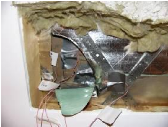
Figure 3.7 – Test cell wall profile showing inside brick surface temperature, outside wrap surface temperature, inside building wrap air temperature and inside plasterboard surface temperature
