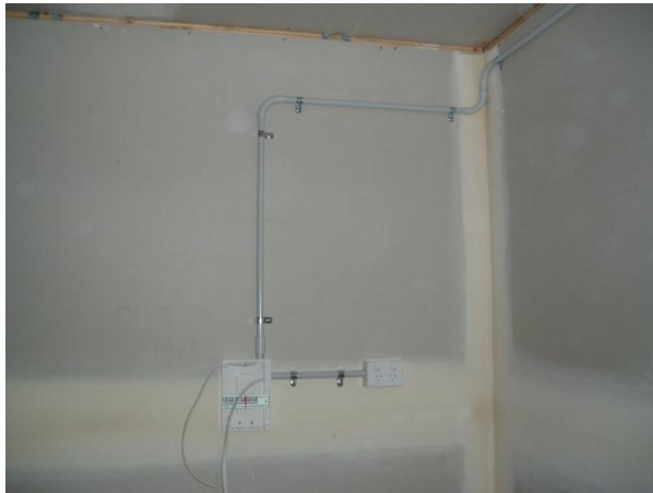
Figure 2.33 - The surface mounting of electrical services
