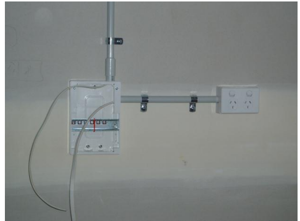
Figure 2.34 - Detail of surface mounted circuit board, conduits and general purpose outlet
