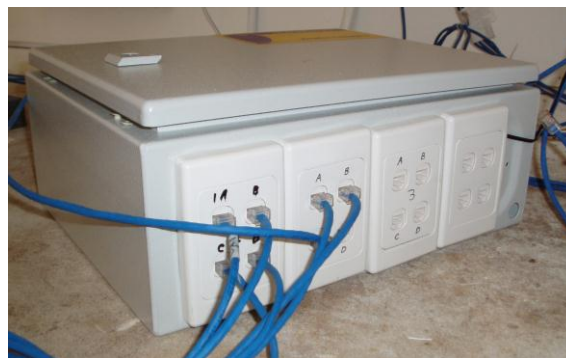
Figure 3.50 - Exterior view of metal box and RJ45 sockets
