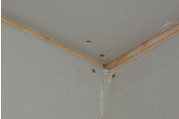
Figure 2.50 - Gap in ceiling corner between wall and ceiling plasterboard
