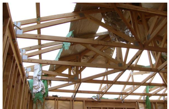
Figure 2.13 - After the storm. Much of the building wrap and roof sarking was removed by strong winds and rain. (July 3, 2006)
