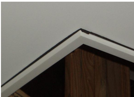
Figure 2.42 - Close up-view of high density foam rubber compressed between prefabricated insert and ceiling
