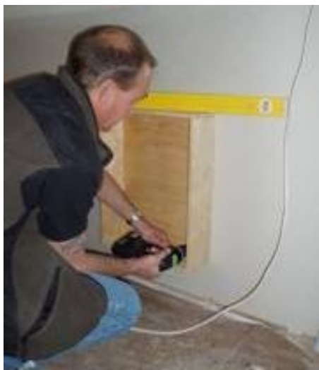
Figure 2.48 - The School technical assistant screw-fixing the heater mounting box to test cell internal wall
