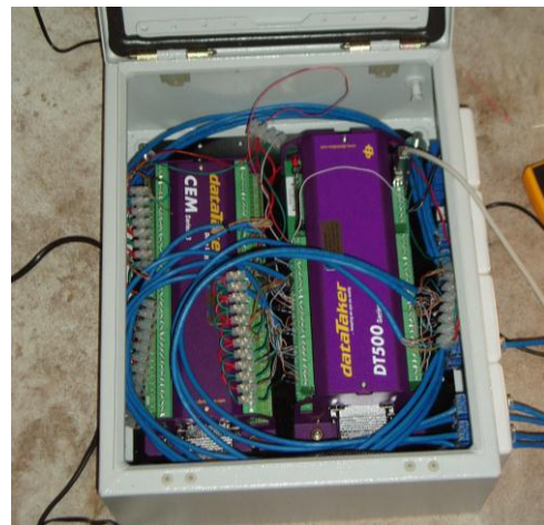
Figure 3.48 - DT500 and channel expansion module in metal case after wiring was installed to RJ45 terminals
