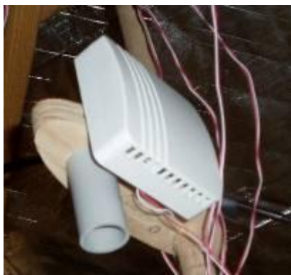
Figure 3.18 – HMW40U relative humidity transmitter installed within a test cell roof space
