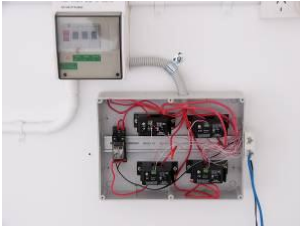
Figure 3.25 – Circuit board enclosure with four SC-551-1 current sensors and heater control relay
