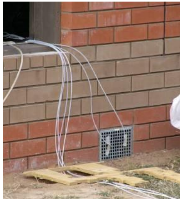
Figure 3.32 – Tracer gas pipes: a dosing gas and a return sampling gas pipe for each zone
