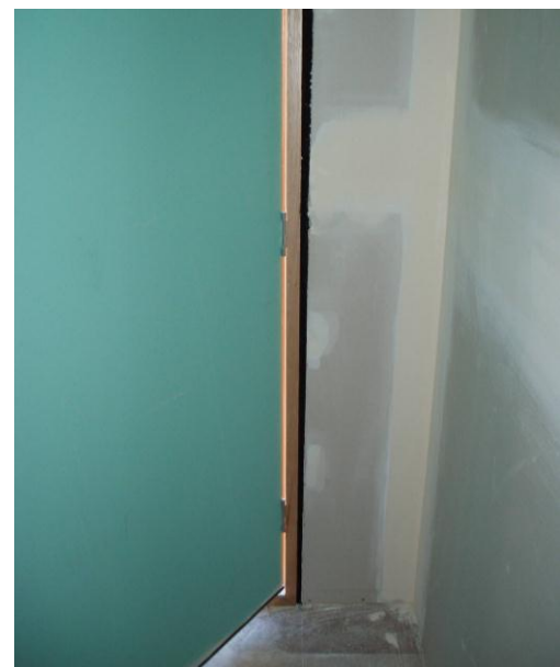
Figure 2.32 - Closed cell foam rubber is installed in gap between door jamb and wall frame
