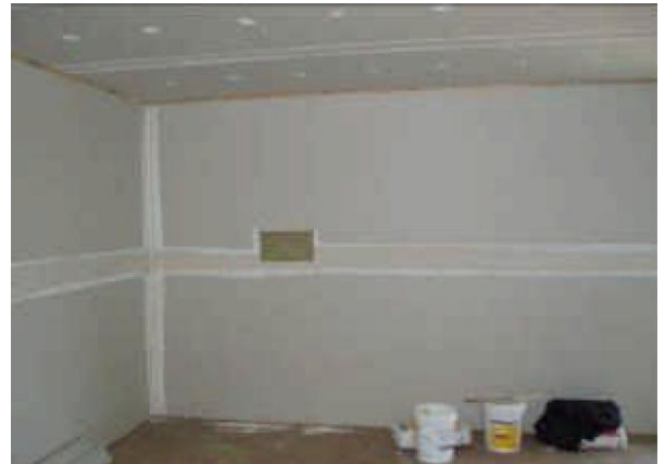
Figure 2.20 – The plasterboard lining has received a plaster shim coat to cover joints and screw fixings (July 12, 2006)
