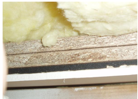
Figure 2.43 - High density foam rubber and particle board sheet affixed to top face of access hatch
