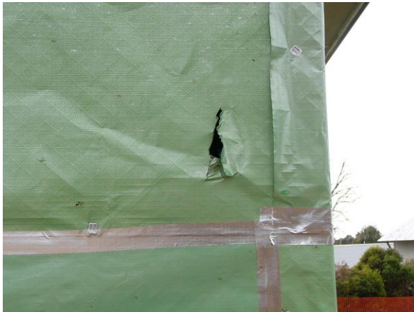
Figure 2.27 - Building wrap torn during construction process
