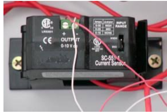
Figure 3.26 – SC-551-1 Current sensor with the electrical cable passing through the sensor and the red and white bell wires connected for the output signal
