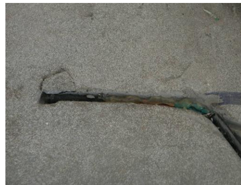
Figure 3.22 - Installing the sensor to the interior surface of the concrete slab-on-ground floor
