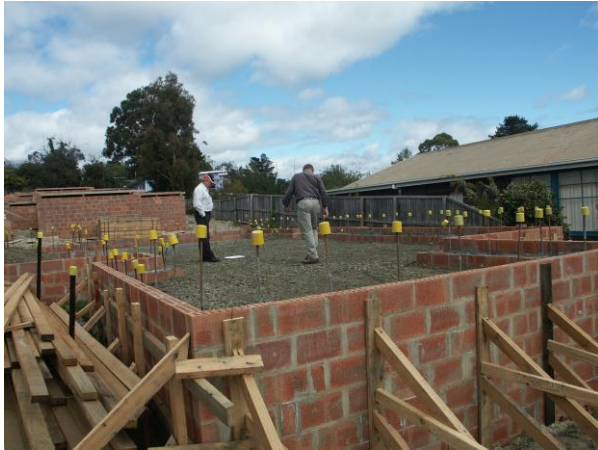
Figure 2.9 – Brick wall and fill preparations for the case study house before concreting
