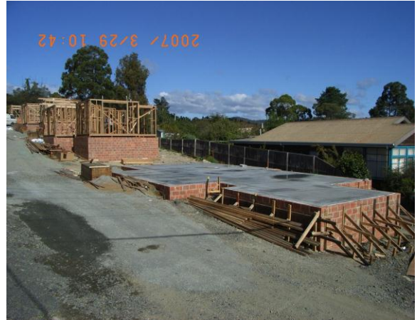
Figure 2.10 - The case study house after the concrete floor has been poured and finished
