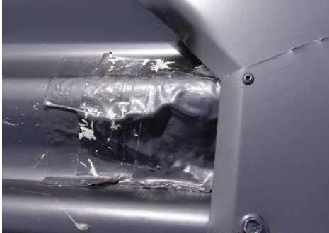
Figure 3.19 - Temperature sensors attached to the exterior surface of the sheet-metal roof
