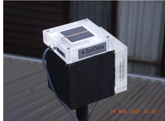
Figure 3.34 - SolData 80SPC pyranometers installed as part of the site weather station
