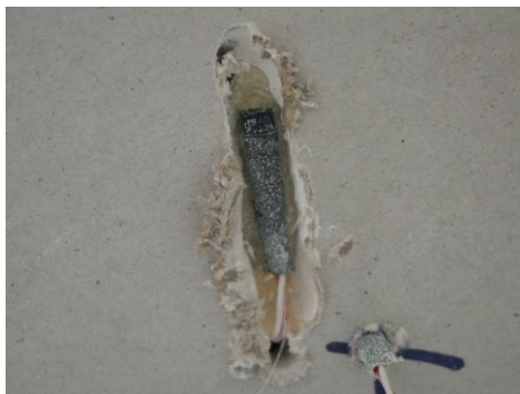
Figure 3.21 - Sensor attached to the inside of paper-faced gypsum plasterboard ceiling before being covered with a very thin layer of plaster
