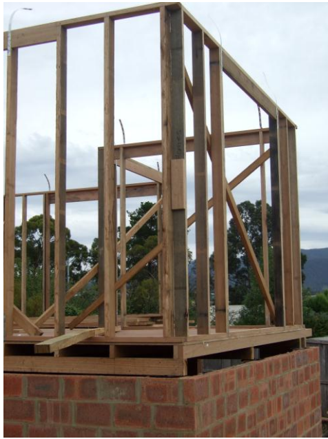
Figure 4.1 - Corner detail at the framing stage of one of the platform floored houses
