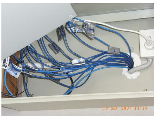
Figure 3.44 - Data cable coming out of wall and connecting to data logger with RJ 45 plugs
