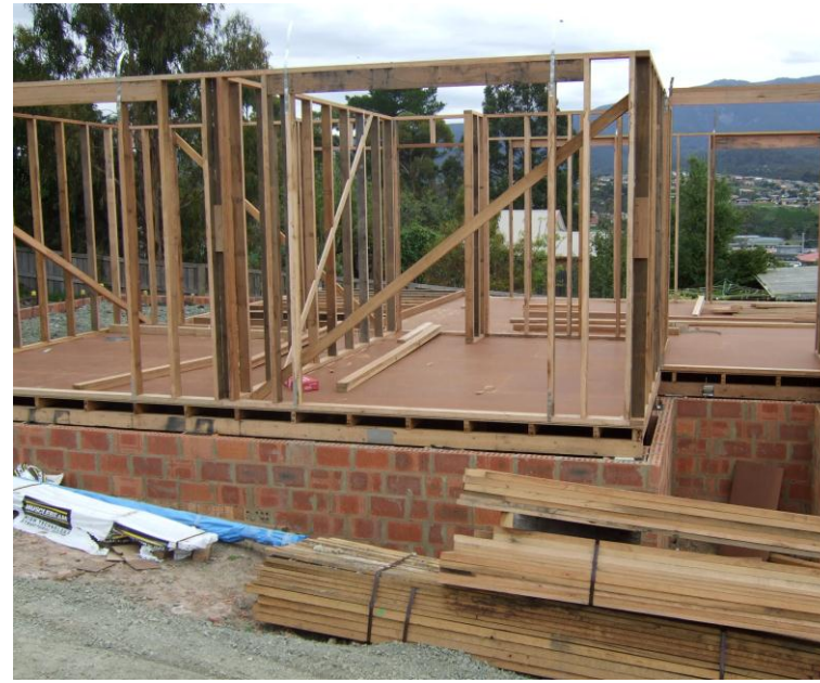
Figure 4.2 - Framing stage of the test house of one of the platform floored houses
