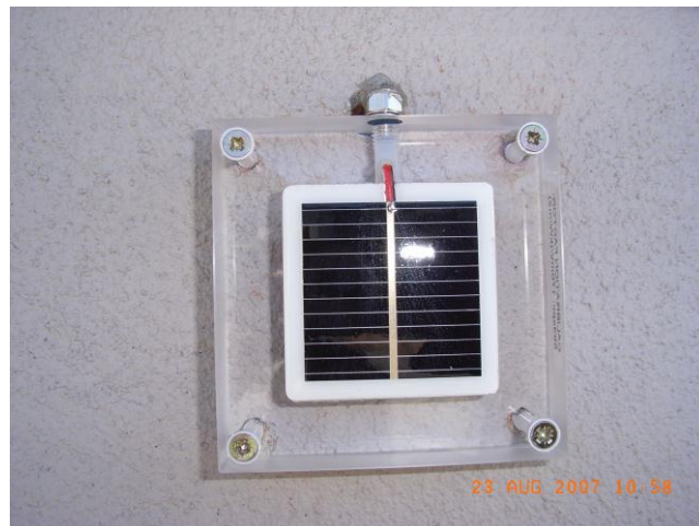
Figure 3.9 - SolData 80 SPC pyranometer fixed external walls of the case study house to measure solar radiation on the wall
