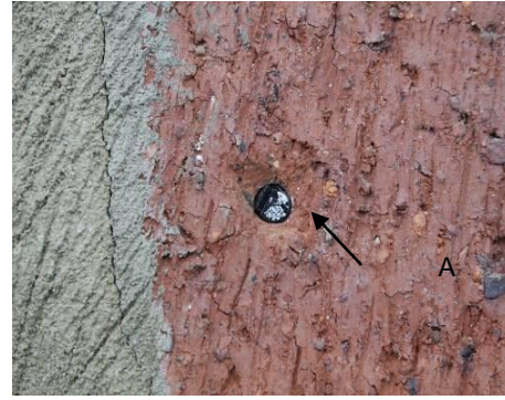
Figure 3.29 - Sensor attached to the outside surface of the brick wall prior to the application of a thin coat of render
