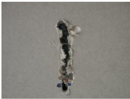
Figure 3.24 – Sensor attached to the inside of the plasterboard wall
