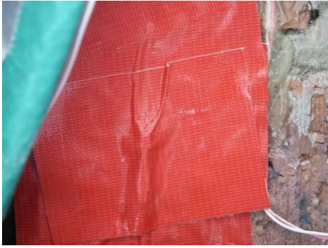
Figure 3.28 - Sensor attached to the inside of the brick wall with red cloth tape
