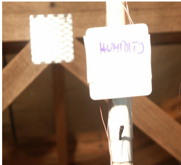
Figure 3.32 - Humidity transmitter installed in the ceiling space
