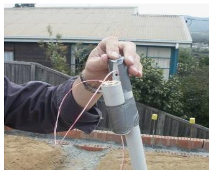
Figure 3.23 - Installing the waterproofed temperature sensor housing for the temperature sensor 1000mm below ground (under concrete slab floor)
