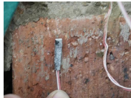
Figure 3.27 – Sensor before being attached to the inside the of brick wall
